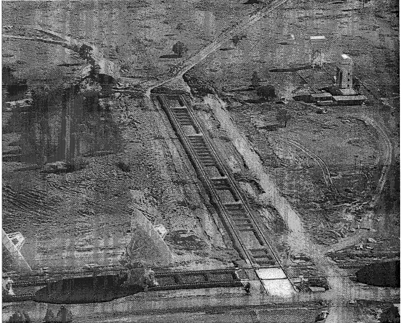
Figure 1: The North Spur of the Compact Array during construction. Photograph by D. McConnell.
