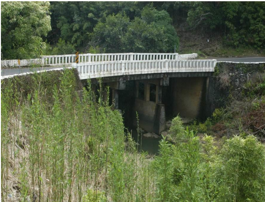
Figure 3. About half the Hāna Belt Road bridges feature a reinforced-concrete parapet of simple vertical balusters and a square concrete rail cap. (Photograph by author.)
