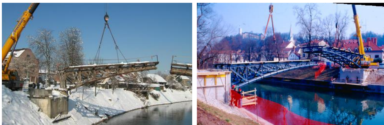
Fig. 9: Dismantling the structure at the second location in 2010 and constructing it again on the third location in 2011 [photos Gruden; Brate].
