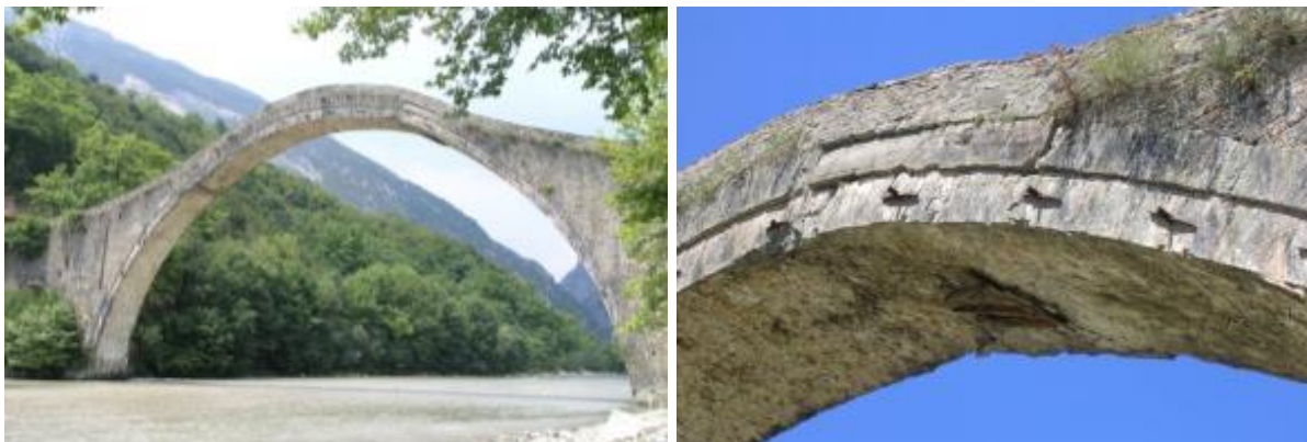
Figure 15: General view of the bridge before the collapse (left) and the area damaged by the explosives (1946) and repaired by reinforced concrete (1947) (right).
