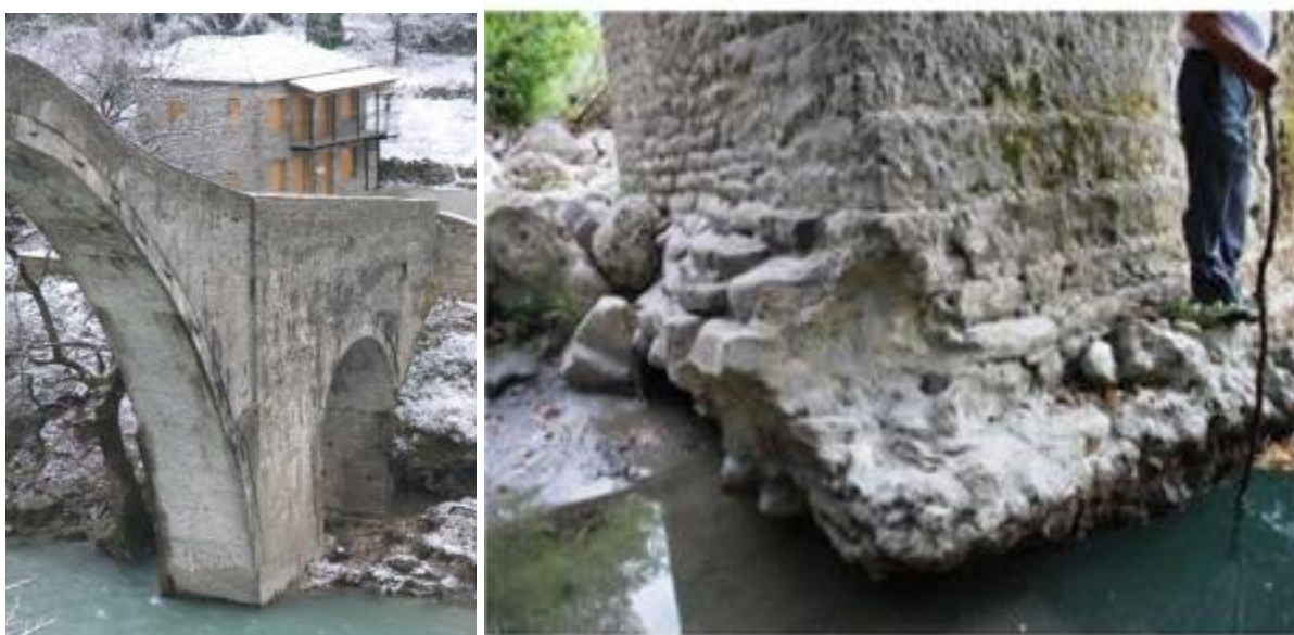
Figure 17: East pier before the collapse (left). Undermining on the foundation of the east mid pier before the collapse (right).
