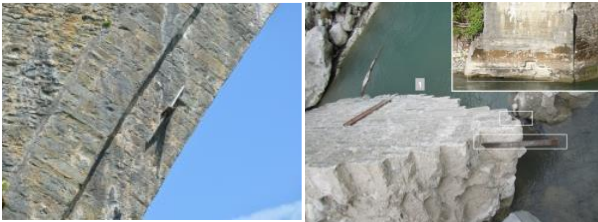
Figure 13: Metal reinforcements: Transversal reinforcement (left), horizontal metal straps in the lower parts of the piers (right).
