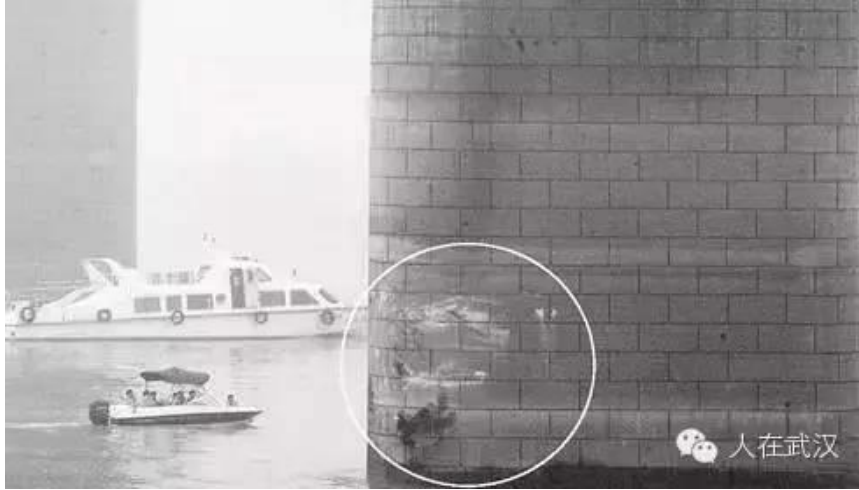
Fig 19. The mark of the Bridge after crush
