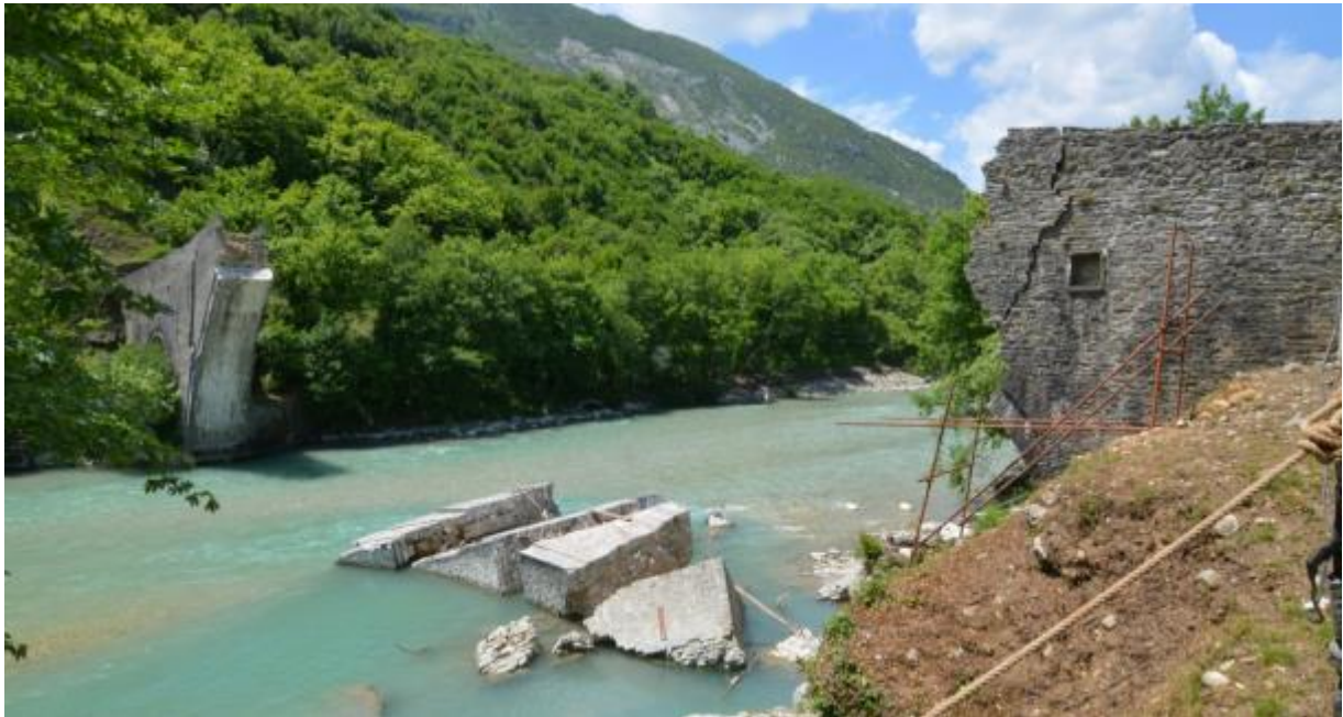
Figure 18: Existing condition of the bridge. The west pier at the left, the fallen fragments and the east pier at the right.
