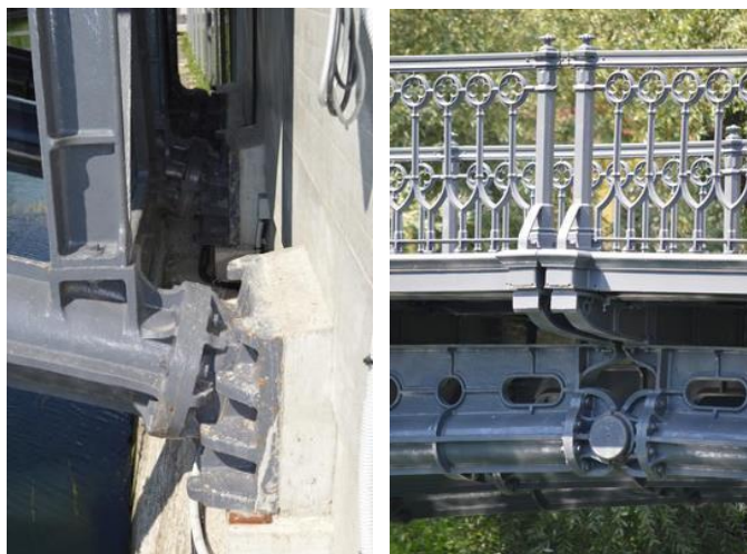
Fig. 12: The hinge at the bridge abutments and the central hinge at the crown of the arch [photo Slivnik].
